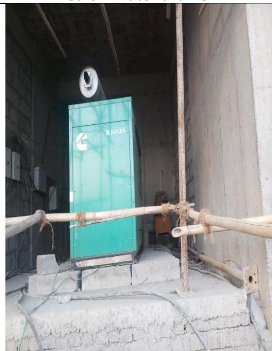
DG sets on site
