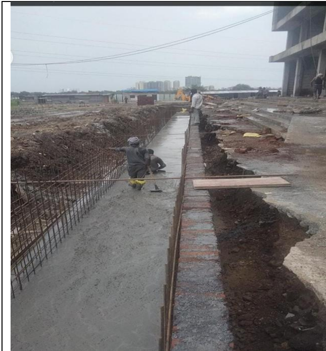
Strom water drains
