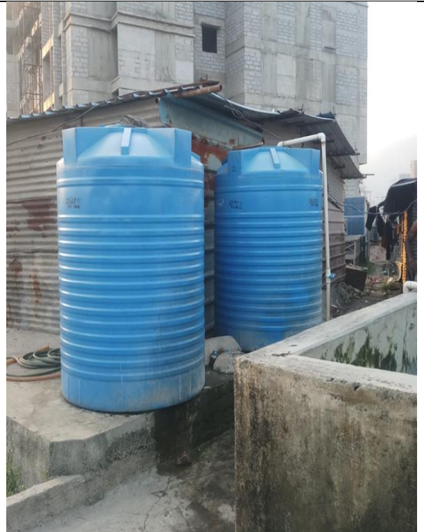
Drinking water tanks
