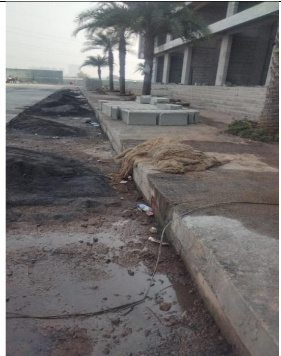
Strom water drains
